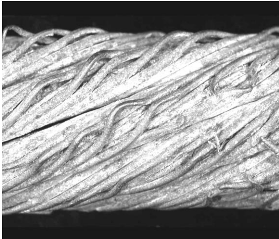
Worn-out or elongated wires of a casting crane rope
